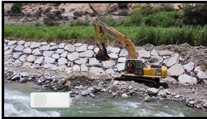
Figura 14: Defensa ribereña enrocado
