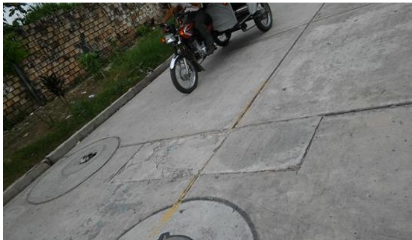
Figura 18: Falla Parcheo(Grande mayor a 0.45m^2 )
