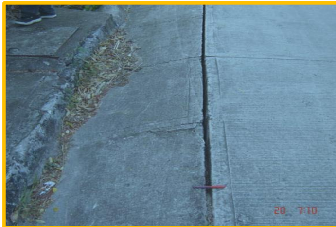
Figura II-19; Desnivel carril berma
