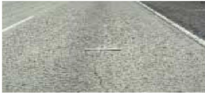
Distress Type CRCP 2 Low Severity Longitudinal Cracking
