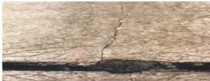
Distress Type CRCP 1 Moderate Severity "D" Cracking at Transverse Crack
