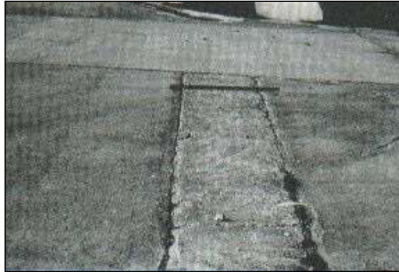
Figura 23, Falla Parcheo Grande (mayor a 45m 2 )
