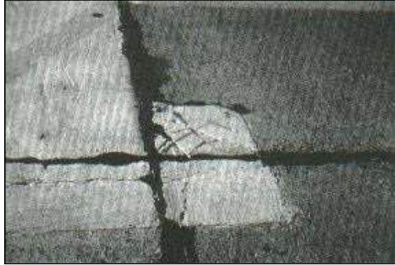
Figura 24, Falla Parche Pequeño (menor a 0.45m 2 )
