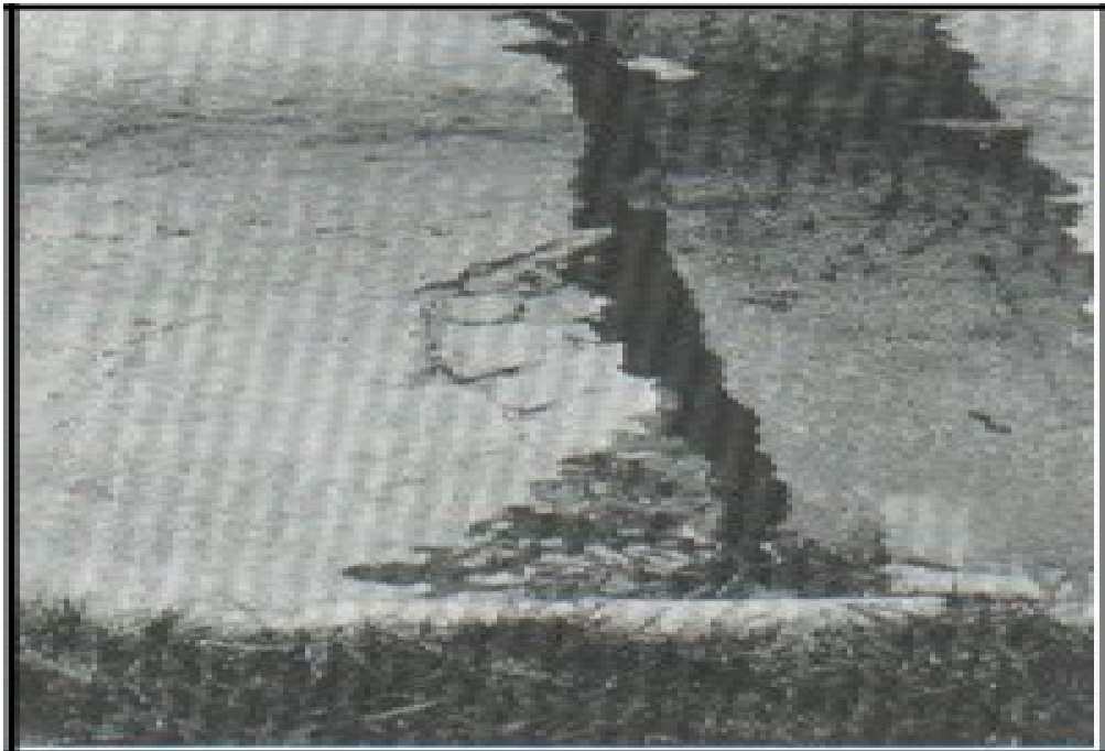
Figura 8: Blowup / Buckling severidad media
